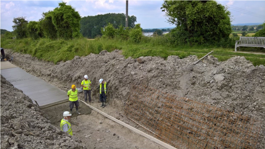
Modern methods to rebuild a traditional canal –Wilstone Reservoir in the distance
