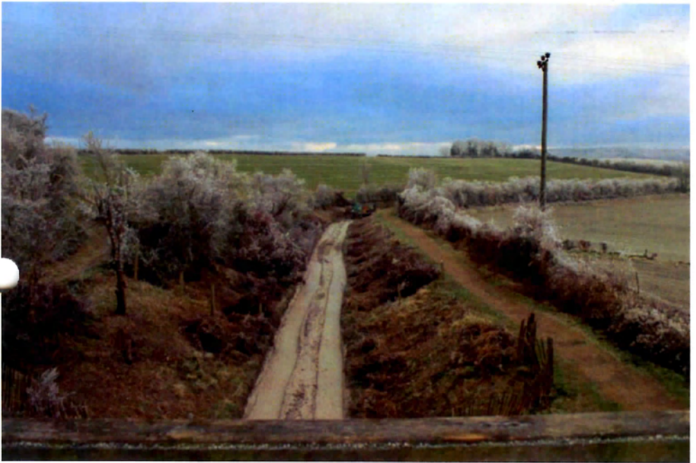
The view from the top of bridge 4A looking back towards Drayton Beauchamp. Pipe capping work can be seen in the distance; December 2010, even the mud was frozen!
