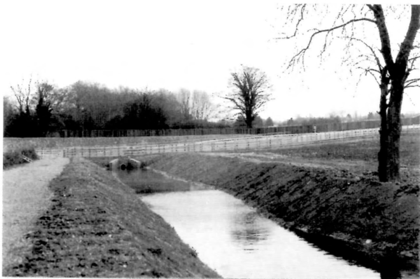
The section of the original line, west of the by-pass, now used to take drainage from the new road. The water emerges from the culvert and flows towards the photographer, i.e. in the reverse direction to previously.
