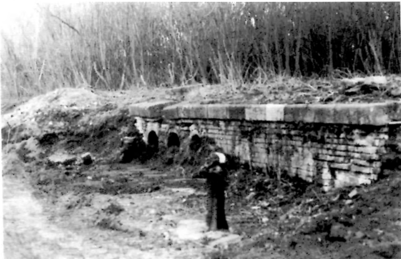
Clearance work at Whitehouses has uncovered this original wharf and culverts. They will be retained as heritage features. The site of the swing bridge is on the left of the view and will be the location of replacement footbridge No.4.
