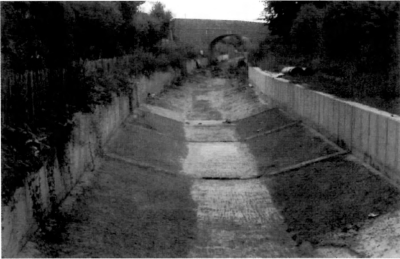
The Bentomat lined section, clearly showing the joints, looking from the stop lock. Only a final dressing of concrete and rubble fill in the centre now remains to be done. A thoroughly professional looking job which is a credit to our volunteer labour force.
