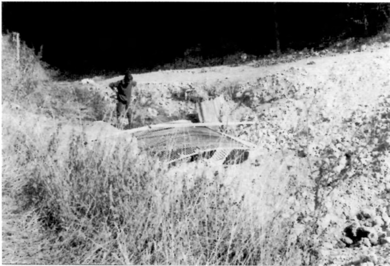
There it was, gone! The site of the former ugly building, now thankfully demolished, over the old sump.
