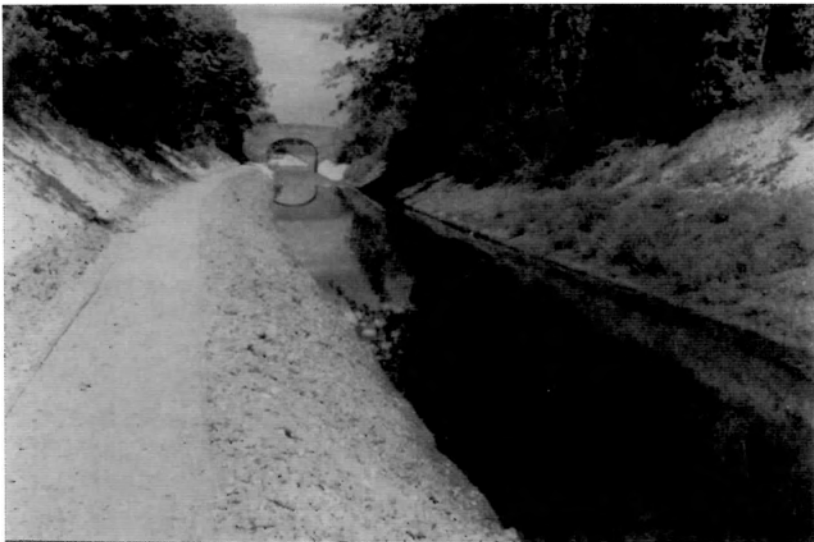
The newly watered section at Drayton Beauchamp, looking towards Drayton Bridge. Although not to navigable depth, the canal certainly looks the part. The edges of the channel are lined with coir rolls until just before the bridge.
