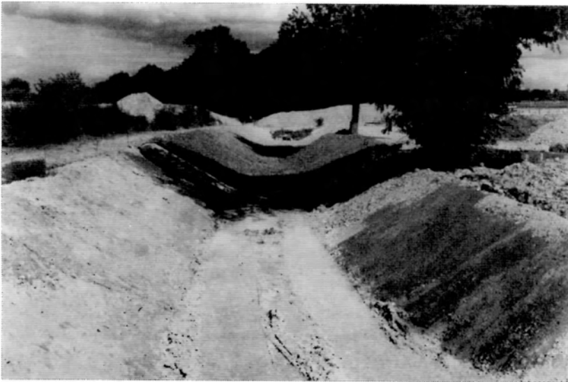
The old line of the canal, on the Buckland side of the new road, relined ready to become the reed bed which will process the road drainage. The direction of flow in this section will be reversed, to flow towards the photographer.
