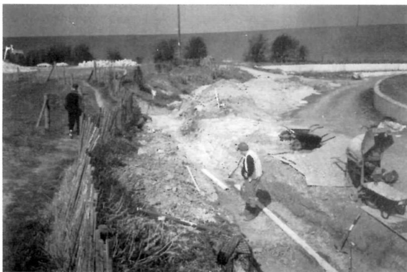
Work in progress on the final length of off-side wall, which will terminate at the white marker just beyond the walker. Apart from the missing short section of wall on the towpath side under the bridge this will complete wall building for Phase I. The off-side beyond this point, to the winding hole will have a soft edge with reed bed.
