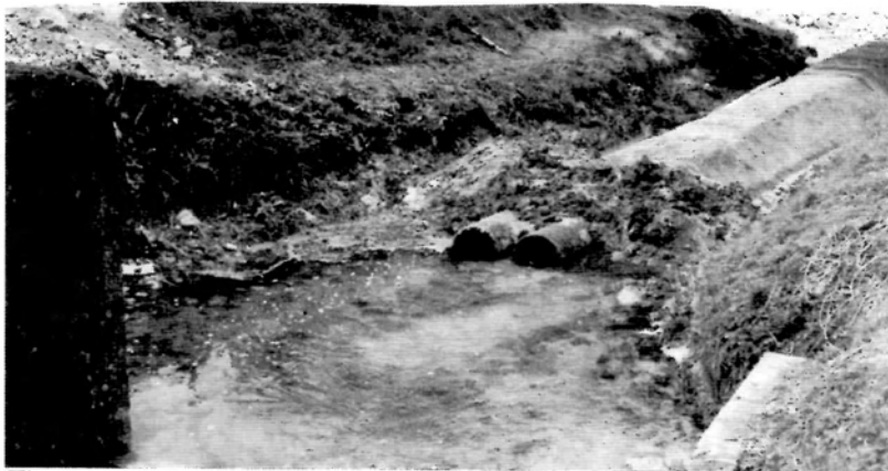
The temporary pipes to take the water under the new road. The old sump, blocked off, is on the left.
