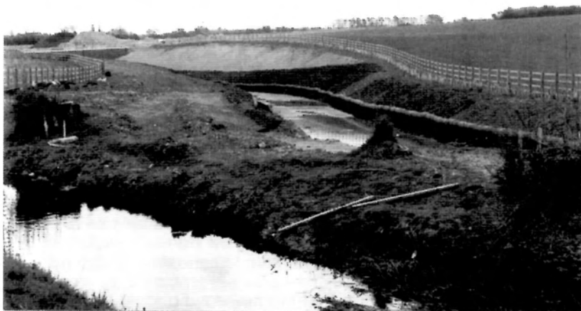
At the western end of the diversion the new channel has been lined; the coir edging can be clearly seen.
