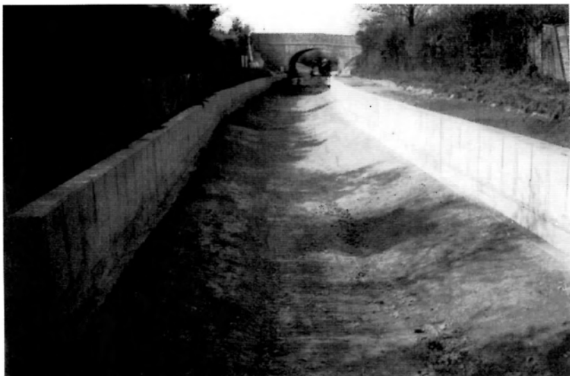
The beautifully excavated and profiled channel between the stop lock and bridge, ready for lining with Bentomat. Note the neat towpath created on the right by backfilling the wall.
