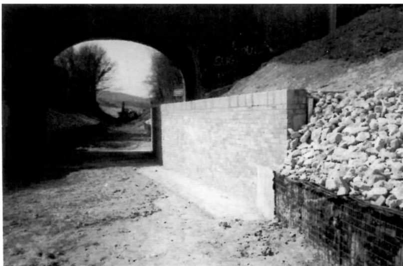
The brick facing used through the bridge hole at Drayton Beauchamp; the bricks match those on the restored wharf.
