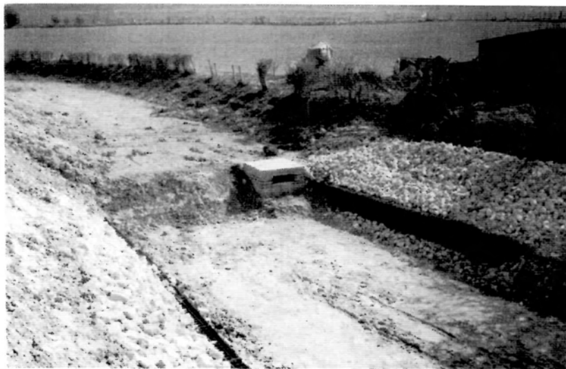
The neat new sump at the eastern end of the reconstructed section at Drayton Beauchamp. The sump will be moved towards Little Tring in stages when Phase II restoration gets underway after 2004.
