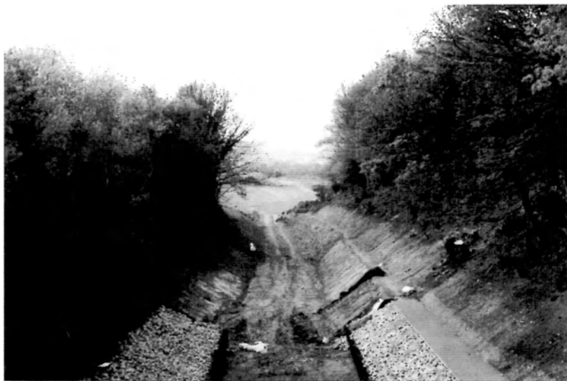
This is the point where the Balfour Beatty section joins British Waterways' newly reconstructed length (in the foreground) at Drayton Beauchamp. One section of lining has already been laid.
