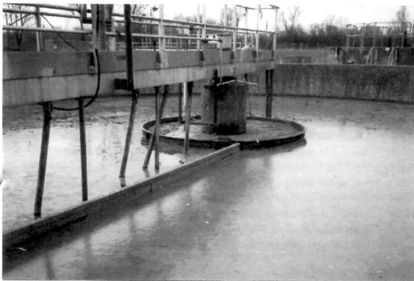
The other key process is the settling tanks; clear effluent weirs over the outside rim, leaving the activated sludge.
