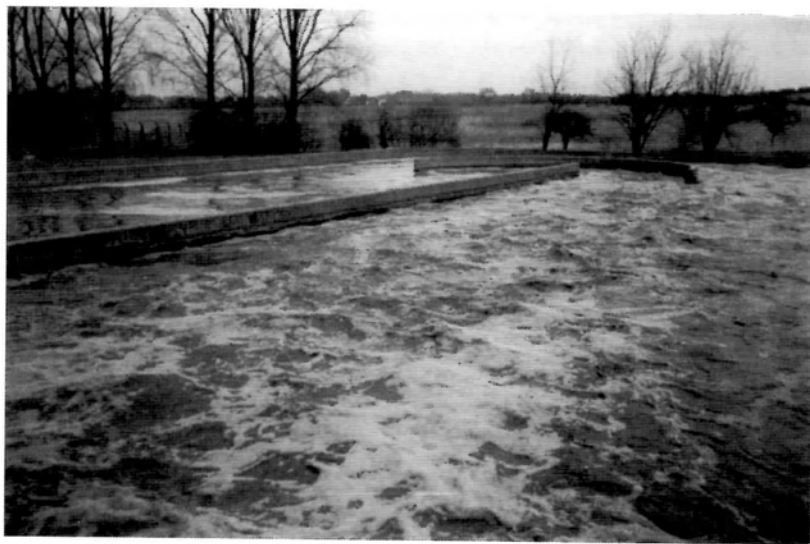
The oxidation whirlpool tank at the heart of the process.
