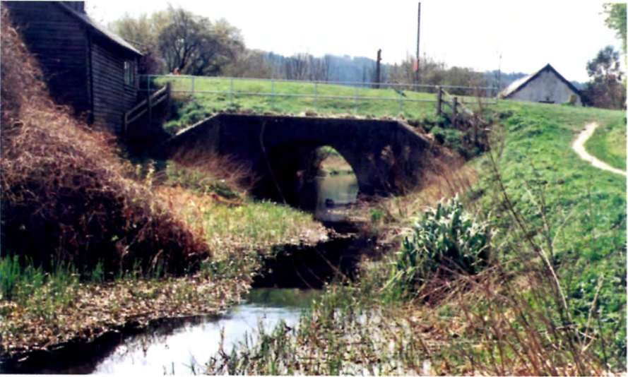
Bridges: The 'large culvert' at Bucklandwharf where a professional study will be necessary to determine what can be done to increase the headroom.
