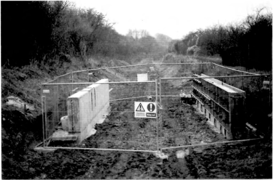
The 'narrows' at bridge 4 well on the way to completion. This view is from the present footpath crossing.
