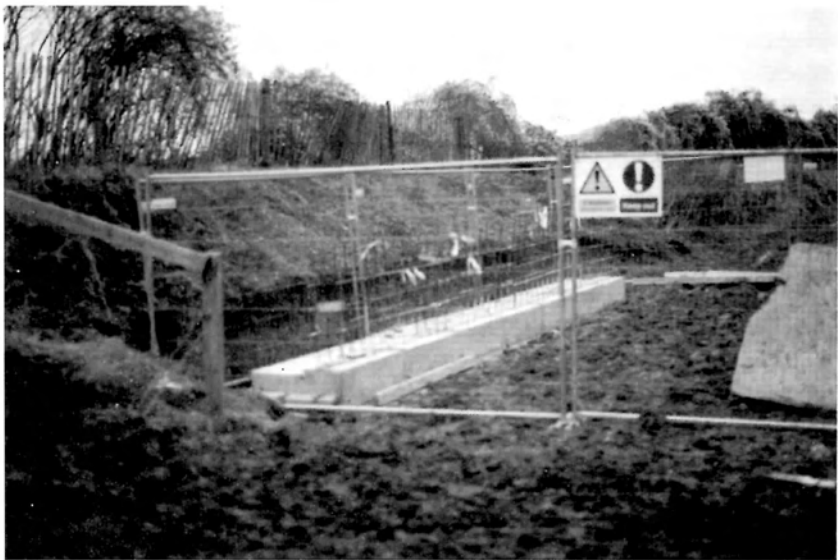
Not so advanced is bridge 4a, although the bases of the walls for the 'narrows' are in place. Again, this view is taken from the current footpath crossing.
