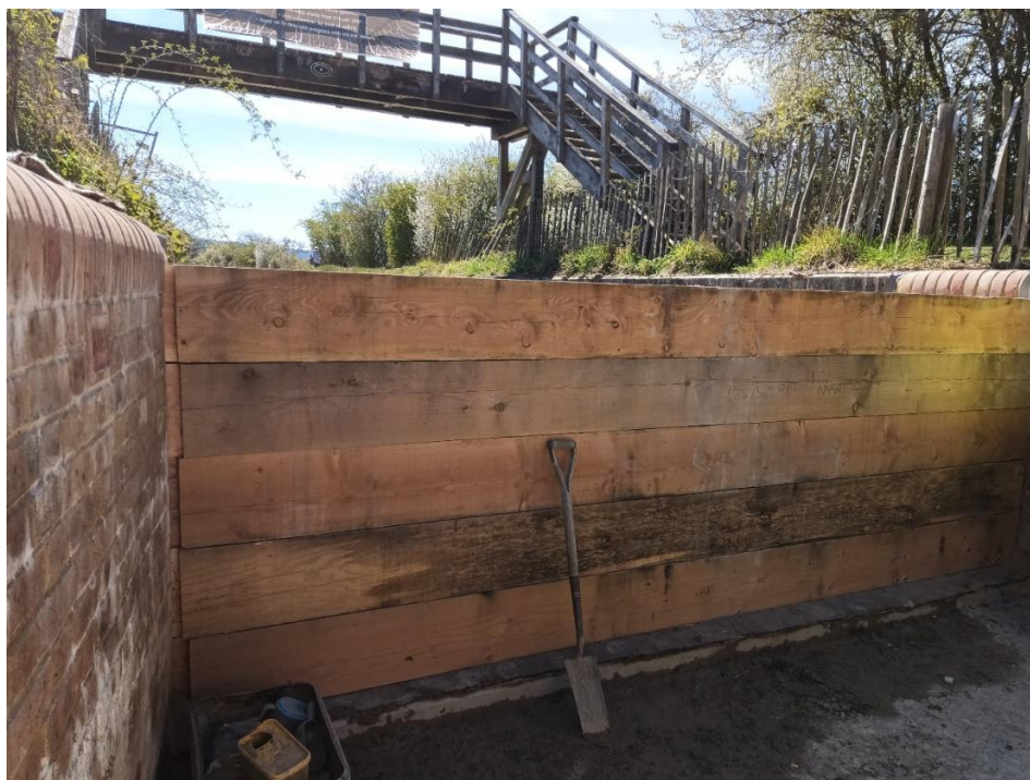
And here are all five planks ready to have Oak wedges put in at each end to hold them in place when under water.
