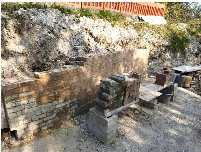
New brick work grafted onto the old. Lime mortar is being used
