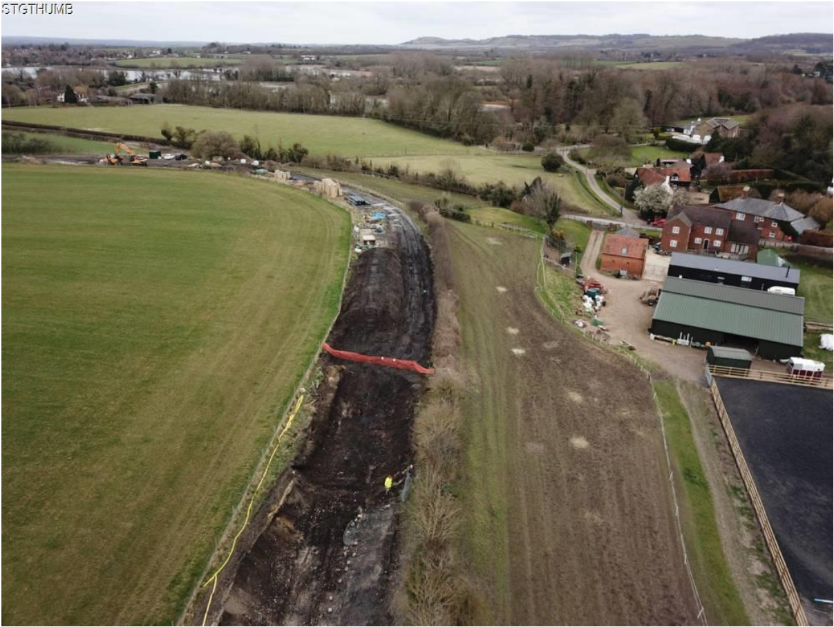
After. The section from the yellow blob (Me!) back to the red fence was excavated. The end of the winding hole is just below the picture edge
