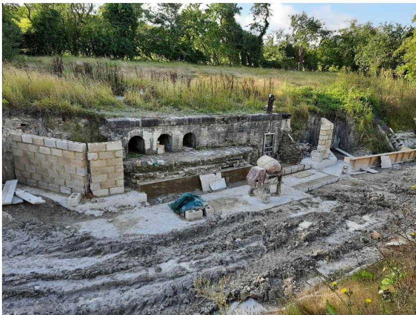
Whitehouses showing completed foundations and block work. The concrete mixer is on the new pipe capping extension. Just next to that are the beams covering the manhole entrance.
