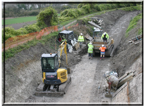
📍 Lining work to prepare for the bund east of bridge 4a, November 14. Photo: Ed
