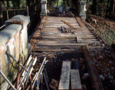
the state of the decking before renewal
