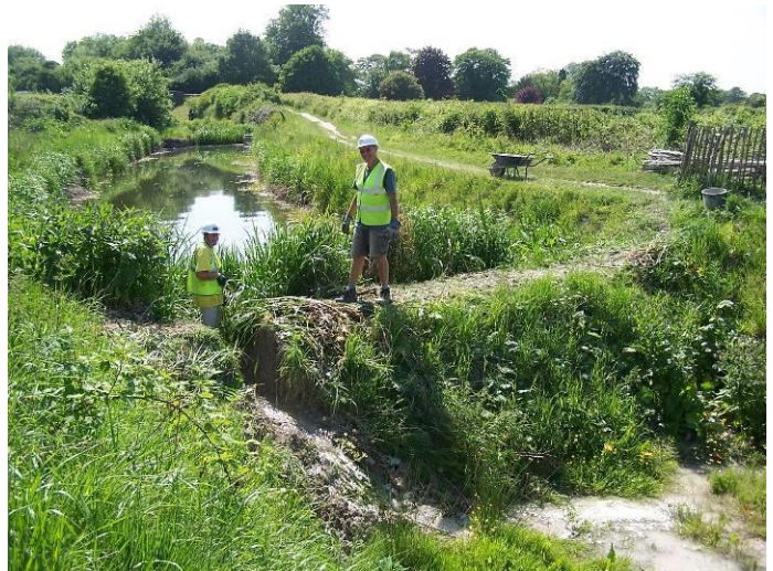
JENNY BRICE AND BOB BARRY BREACH THE BUND AT THE END OF THE FIRST 60m TO RE-WATER STAGE 1
