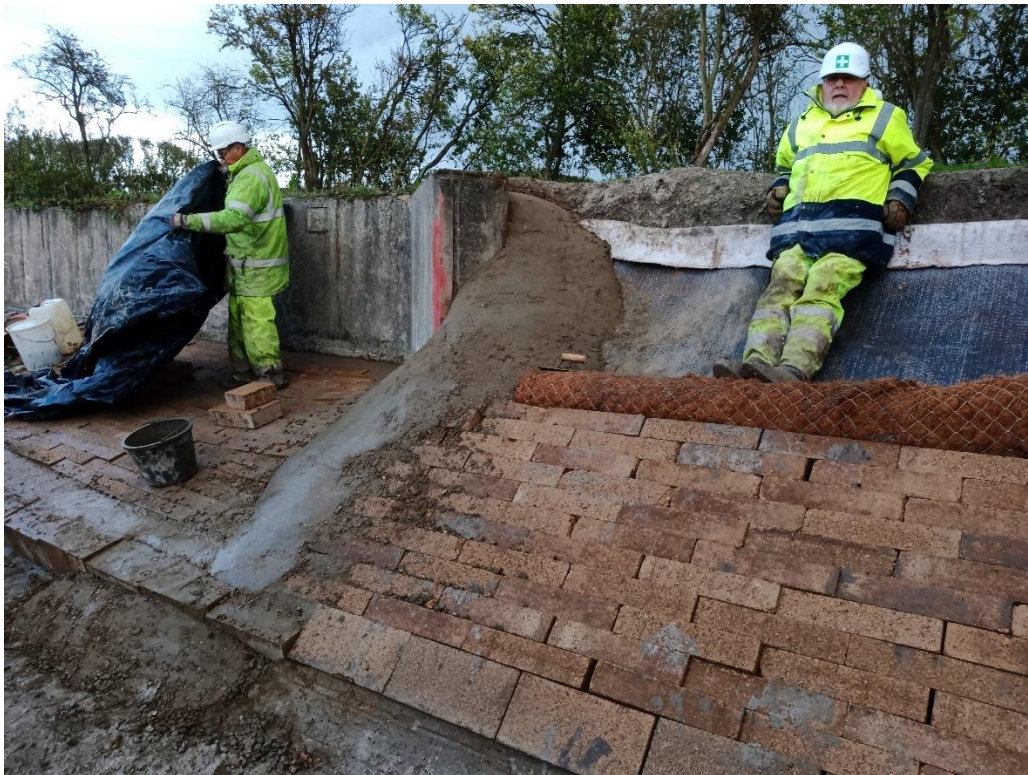
The last part of the concrete join infill. (not much more to do Peter!)
