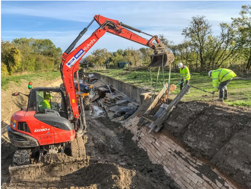
The backfilling frame being moved to the next section. Early morning sun not helping! (photo Tony Borrill)
