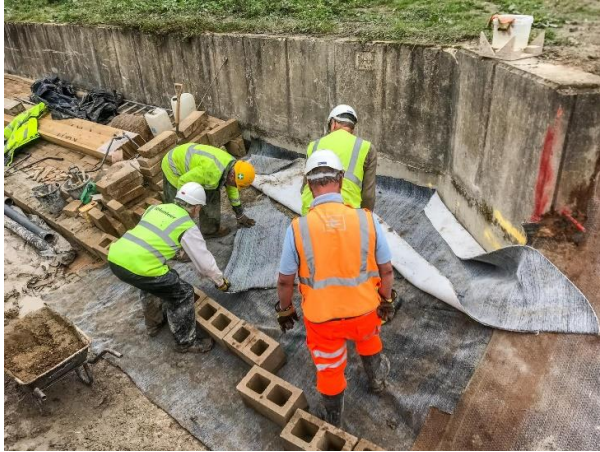
Last part of Mooring wall, Bentomat being tailored to fit (Photo Tony Borrill)
