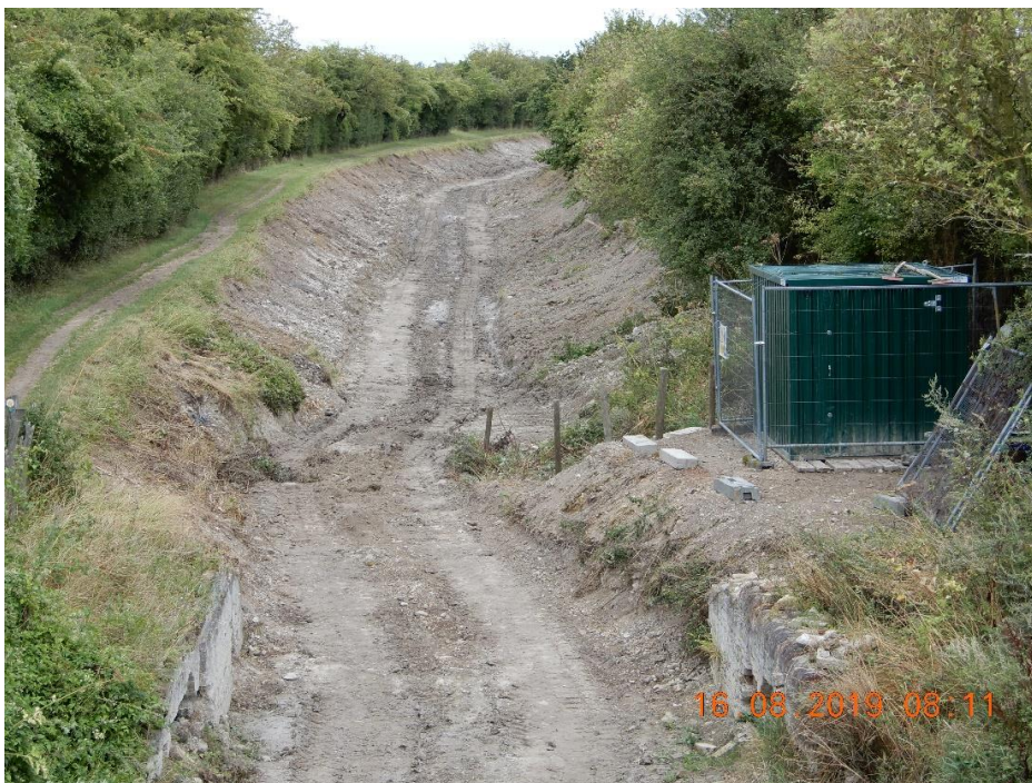
View from Bridge 4 looking towards Little Tring. The bank has been marked out and vegetation clearance and bulk excavation started
